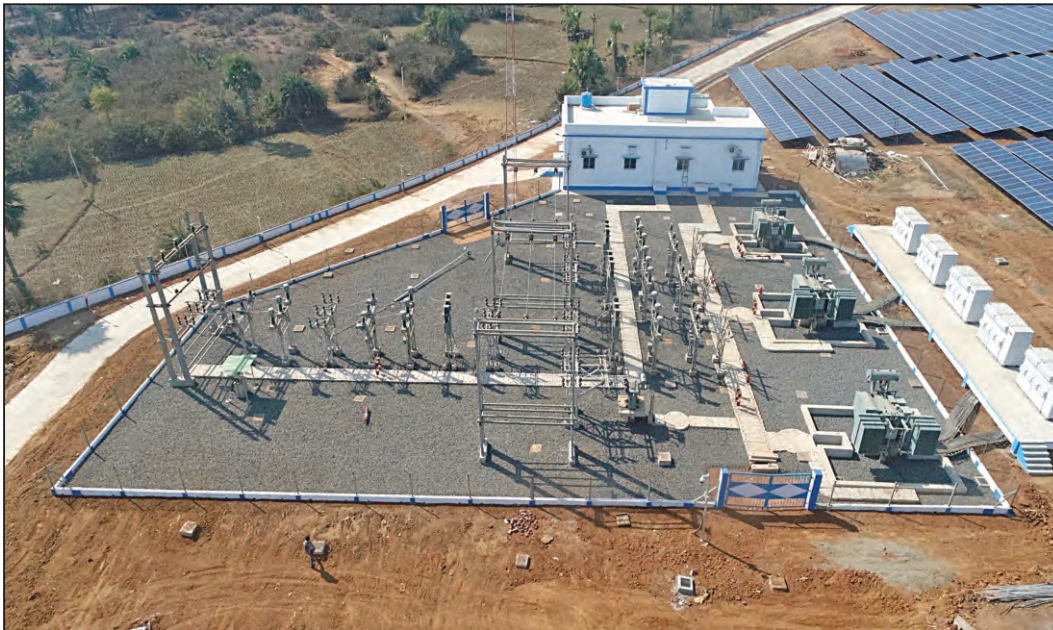
10 MW Solar Power Plant-Dhaka-1
